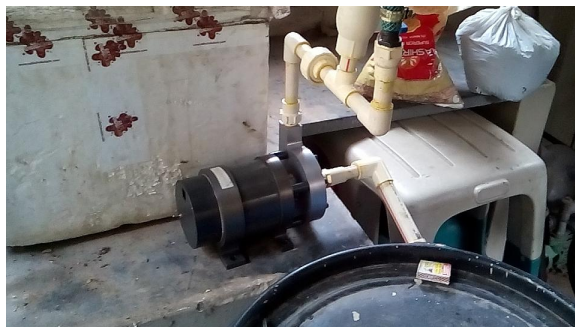
300 W pump in operation
